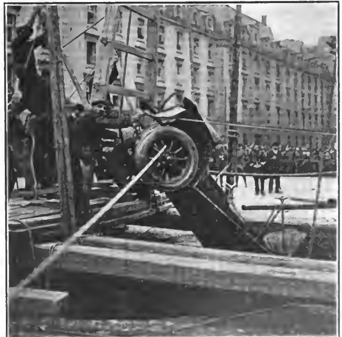
In a recent cave-in of a street in Paris a taxicab was carried into the hole. The illustration shows the removal of the wreck
